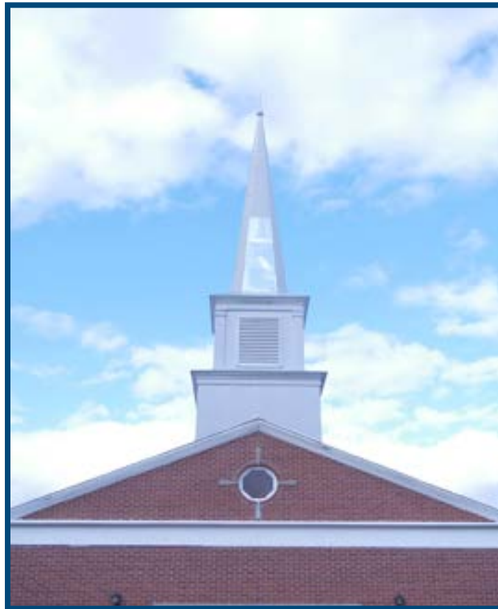
The repaired Tabernacle steeple. In time, oxidation will make sure the repaired portion will match the rest of the steeple.
